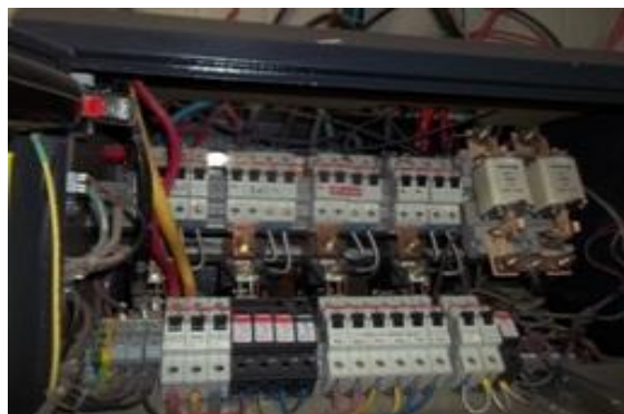
Figure1: Rectifier equipment at BTS site
