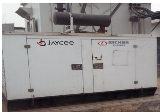
Figure7: DG set for a BTS site
