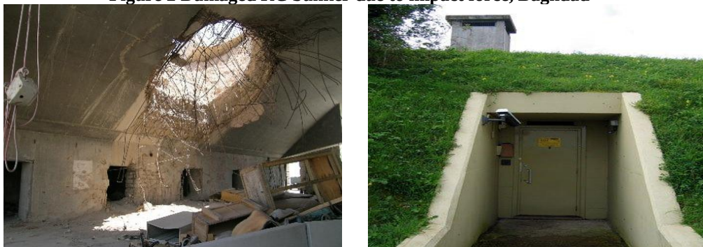
Figure 2 Damaged RC bunker due to impact force, Baghdad
